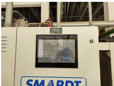
Figura 13: Painel do chiller.
